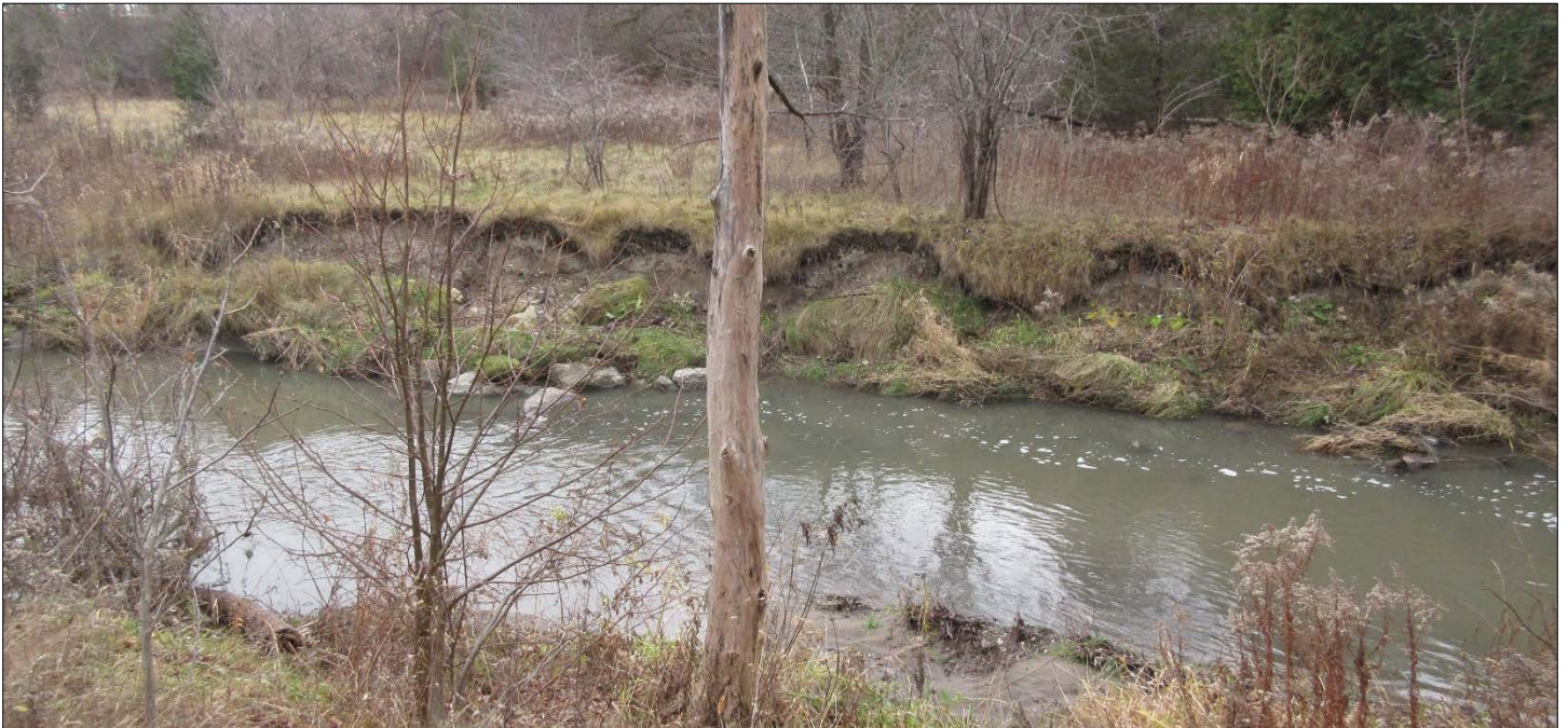
Figure 3. Current conditions at Site I-149, with view of eroding banks. Source: TRCA, 2018.
