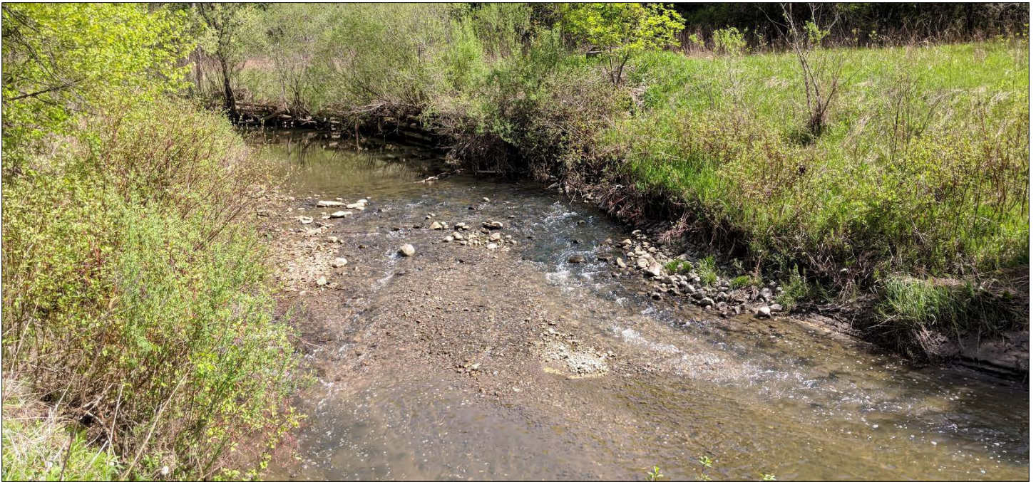
Figure 2. Current conditions at Site P-070, with view of existing cribwall on east bank. Source: TRCA, 2018.
